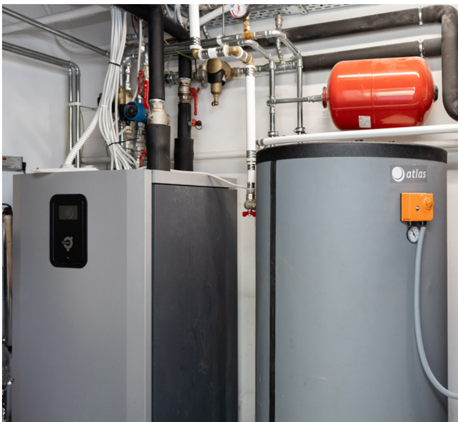
Thermia Mega S (14-42 kW) in the machinery room
